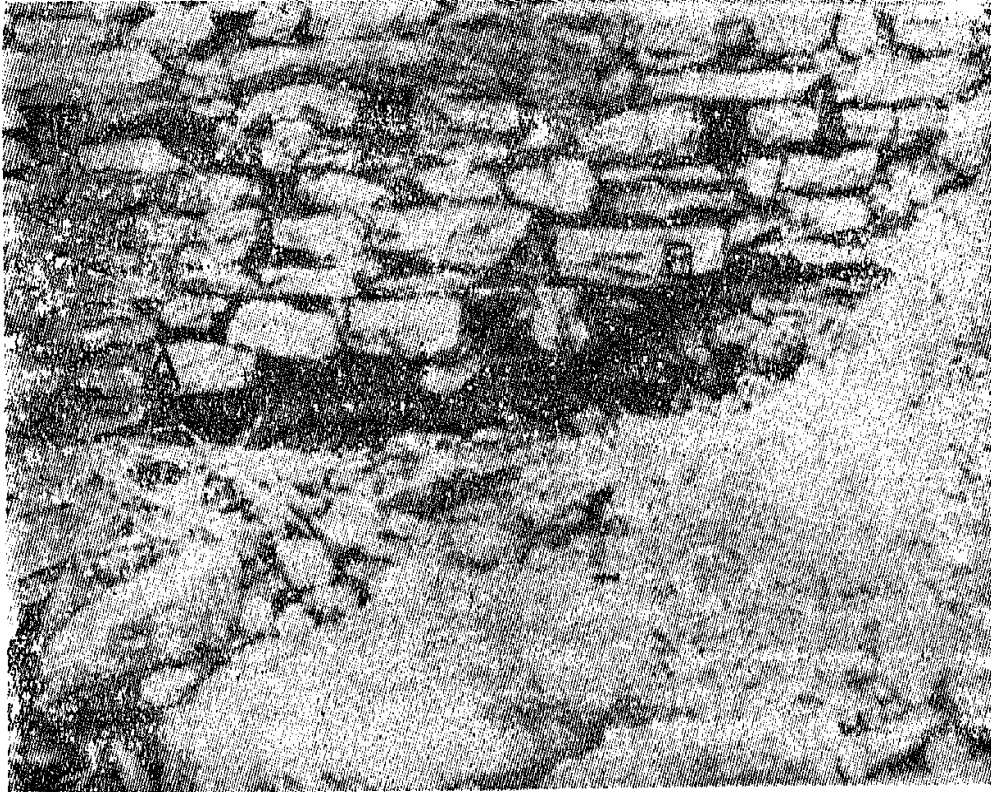
Photo—1. Loss of stones and formation of pockets in retaining wall because of water erosion
