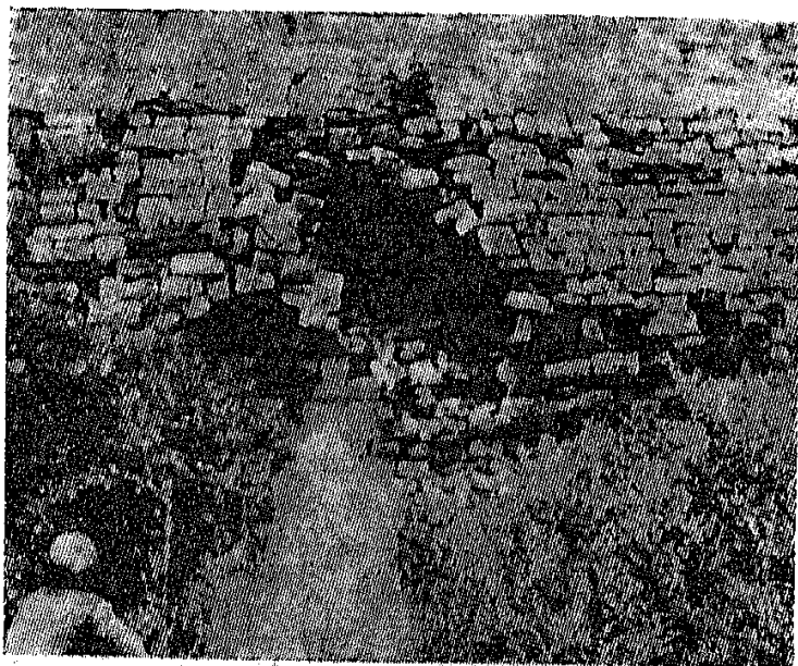
Photo 4. A retaining wall subjected to bulging and loss of stones
